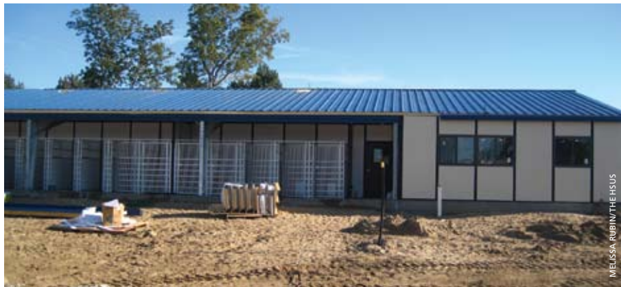
The Houndquarters building and new play area offer dogs plenty of room to roam; they can access exercise space through doggie doors in their kennels. They won't get muddy paws, once the grass starts growing.
